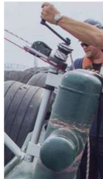
Image E6 The bitt dome top was welded on. Weld will be cleaned up where the davit will sit *7 Series shown – 3 Series mounting is identical*
